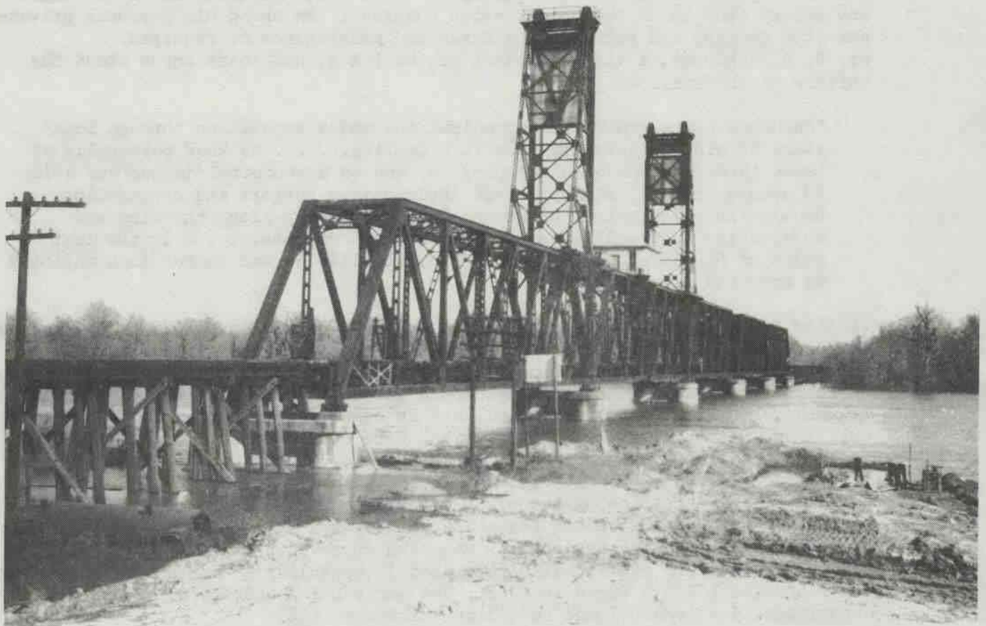
Lift span over the Black River at Jonesville, Louisiana, on the Packton-Vidalia line. This was a major structure for the L & A, with a total length of 840 feet in the five spans. The view is toward the east. The bridge opening in September 1913 enabled through service from Shreveport to Natchez, Mississippi. (Author's collection)
