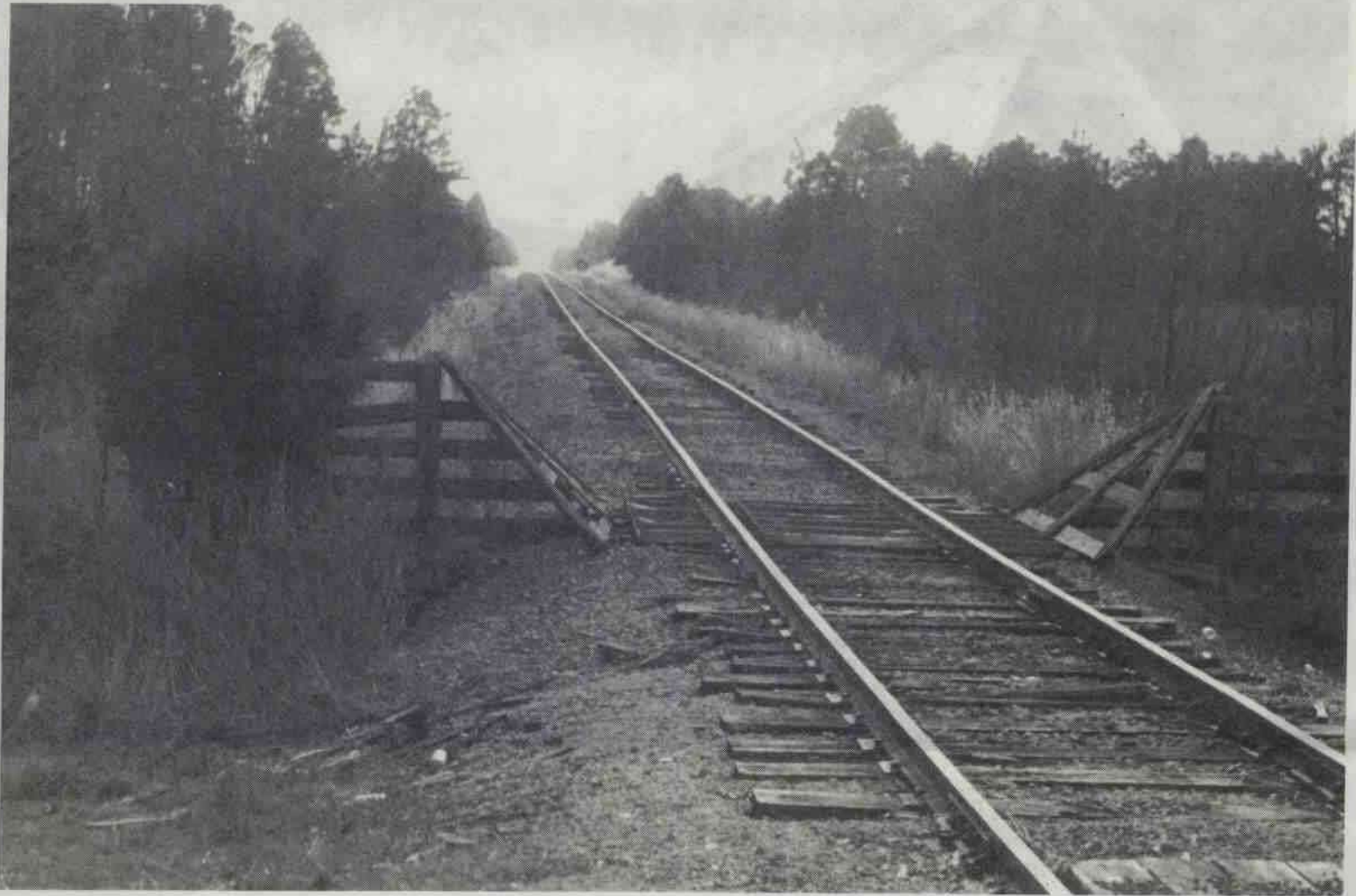
Looking south, the Louisiana & Arkansas RR cattleguard on the Texas sub-division between Newsome & Pickton, Texas on the service track into the old Tidewater Refinery Works. (December 29, 1987 photo by Bill B. Bailey)
